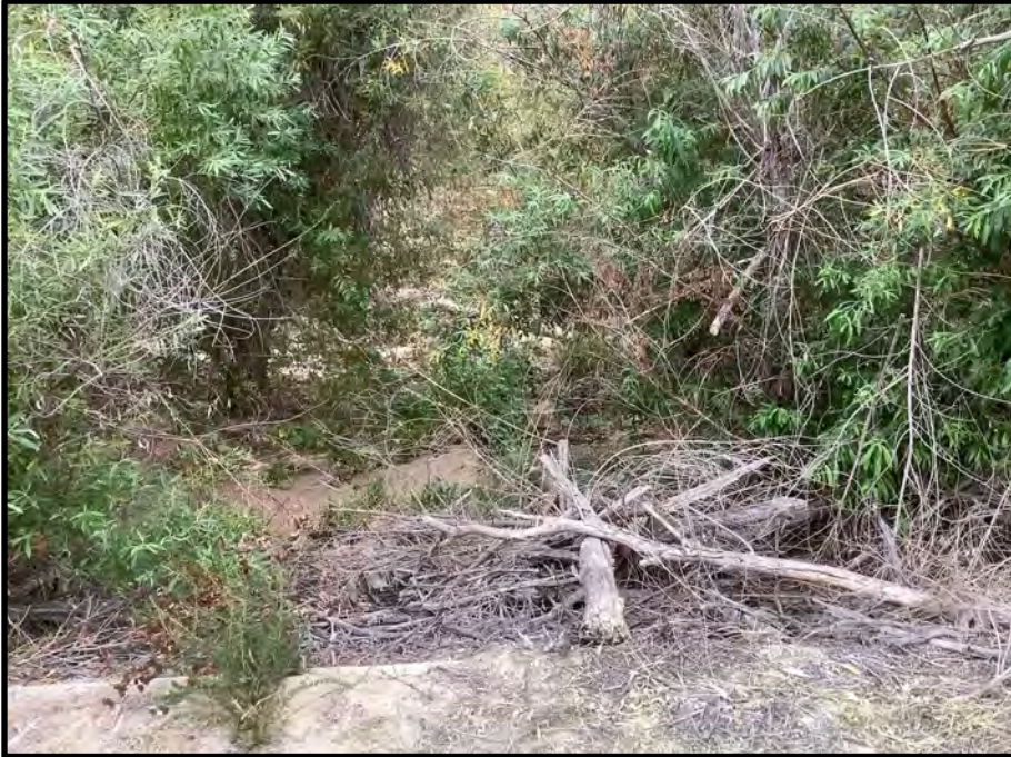
← Blockage prior to removal 11/7/23.
