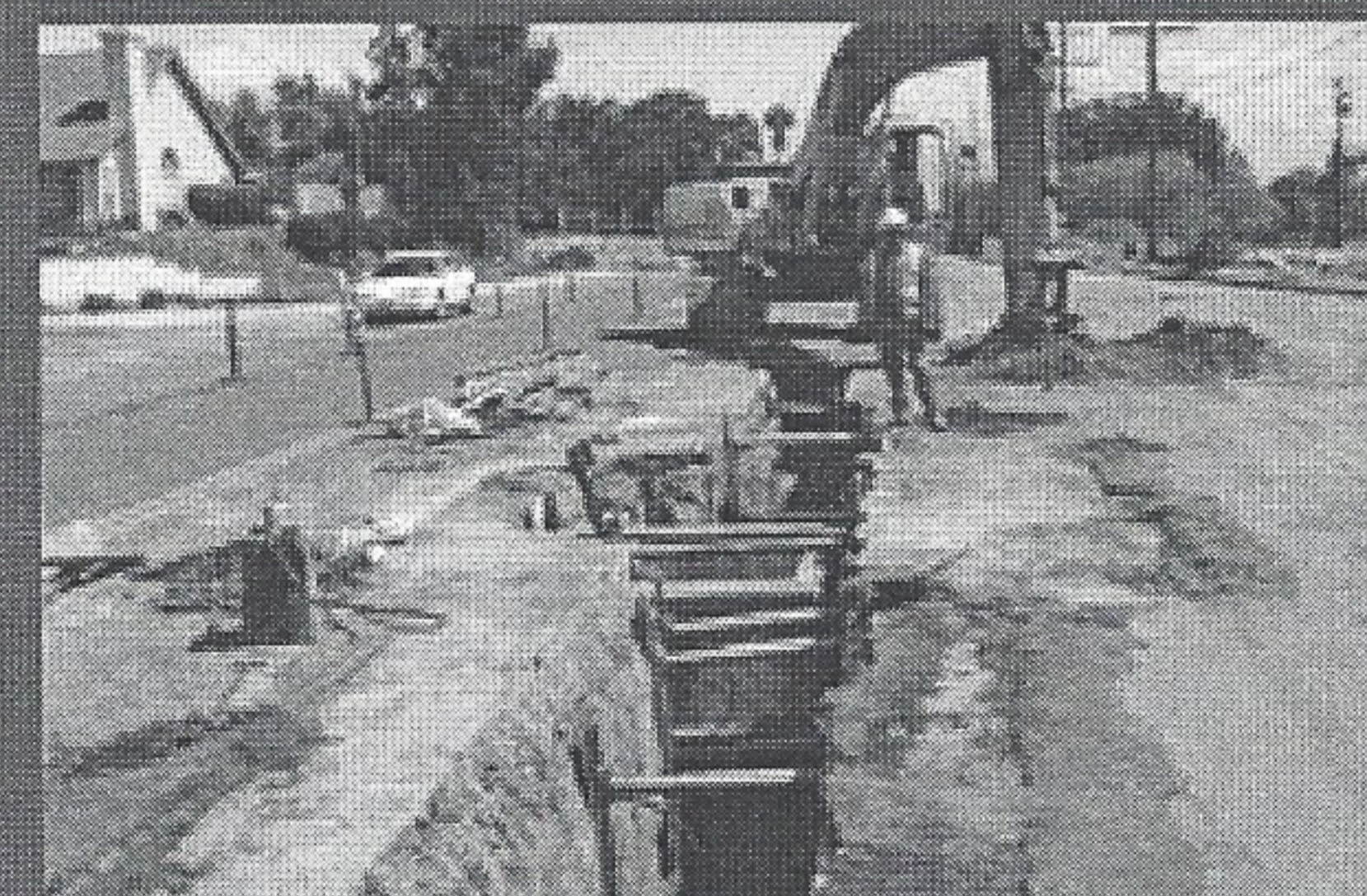
Washington Ave. Sewer - Palomar Rd. View of force main sewer pipe trench in Palomar Rd. southeast of Clinton Keith Rd.
