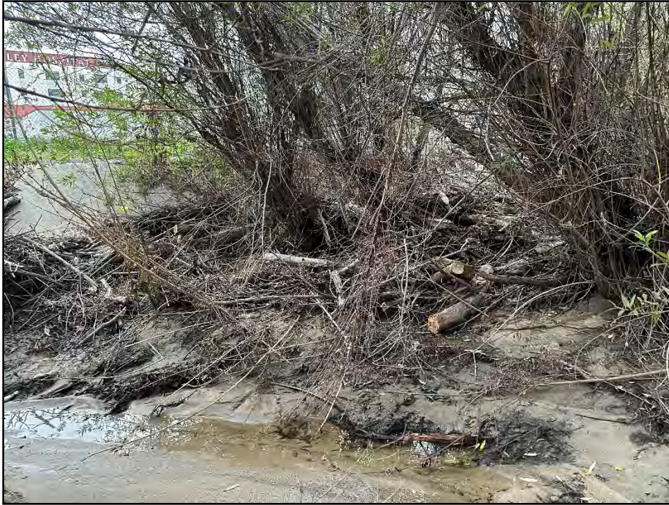
← Blockage prior to removal 12/29/22.
