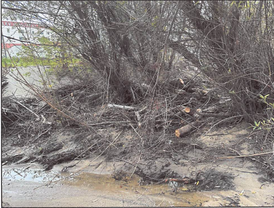
← Blockage prior to removal 12/29/22.
